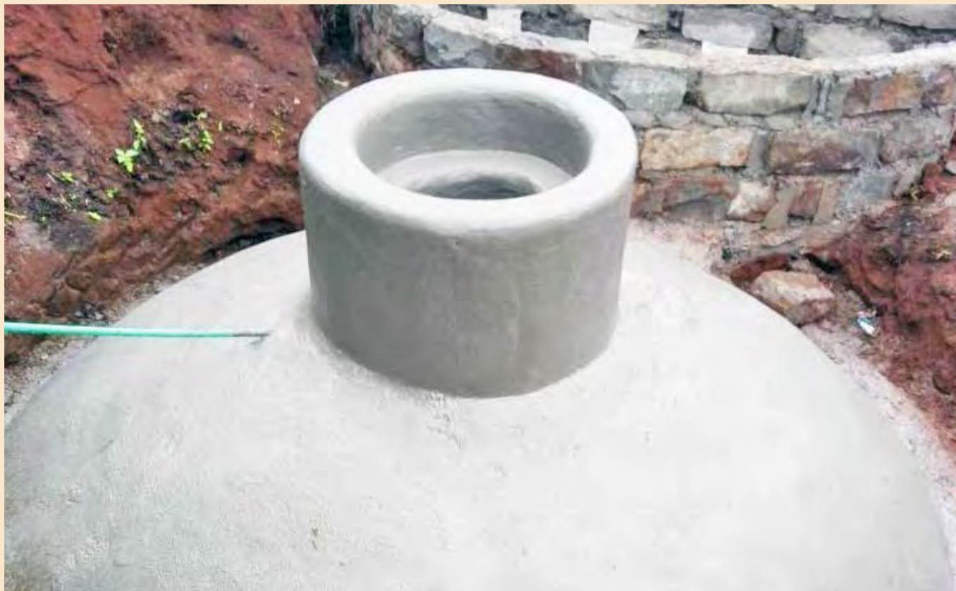
Photo: Blueflame Water and Energy Solutions
