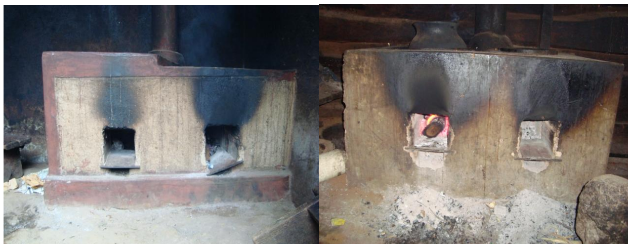
Figure 4: Examples of Okoa stoves with poorly constructed ash trays resulted into black stains (soot) on their front view.
